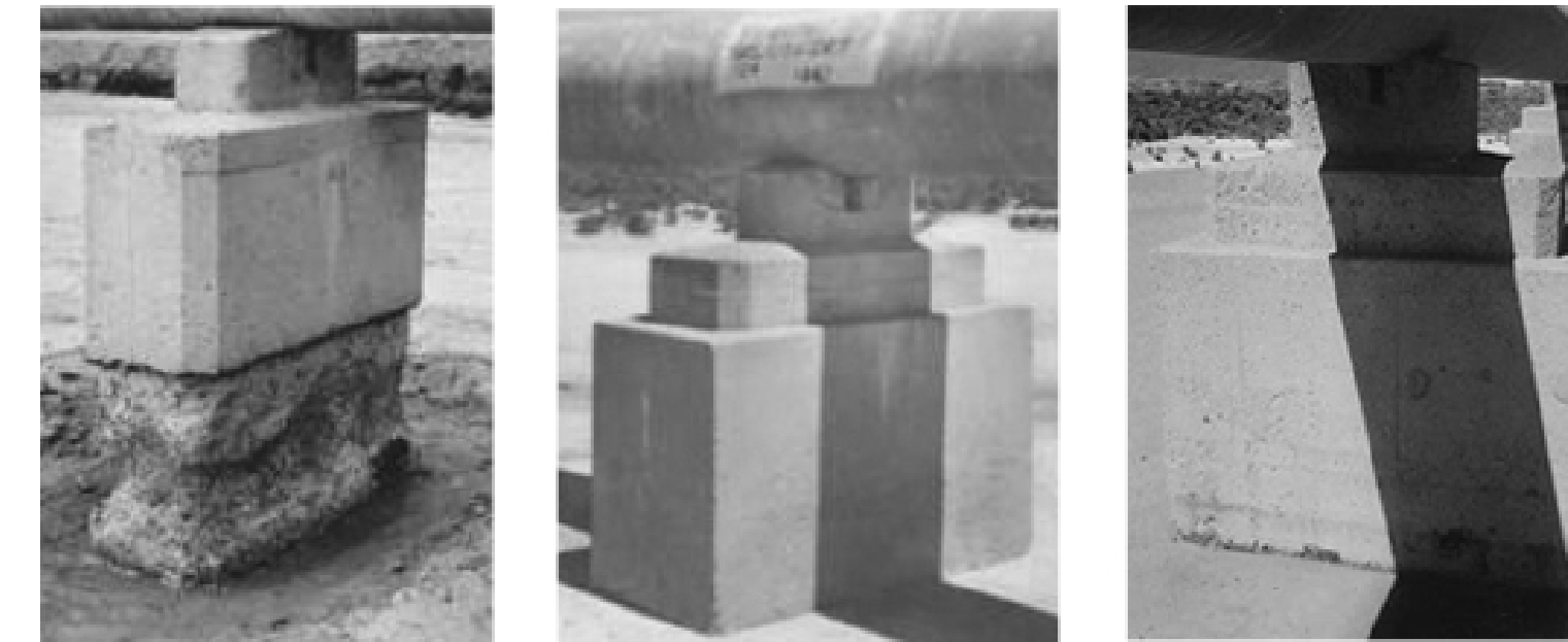
20 year old traditional concrete Lightly reinforced calcite concrete Same calcite concrete after 50 years
