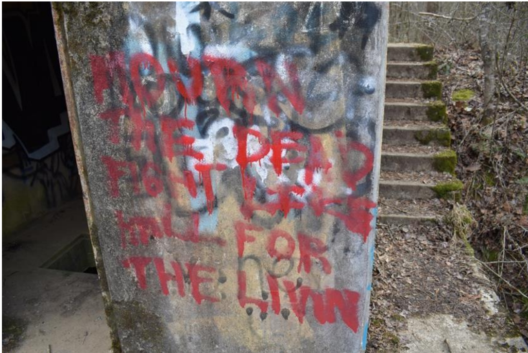
Figure 3. An example of graffiti from the pump station at the former GNAL site.
