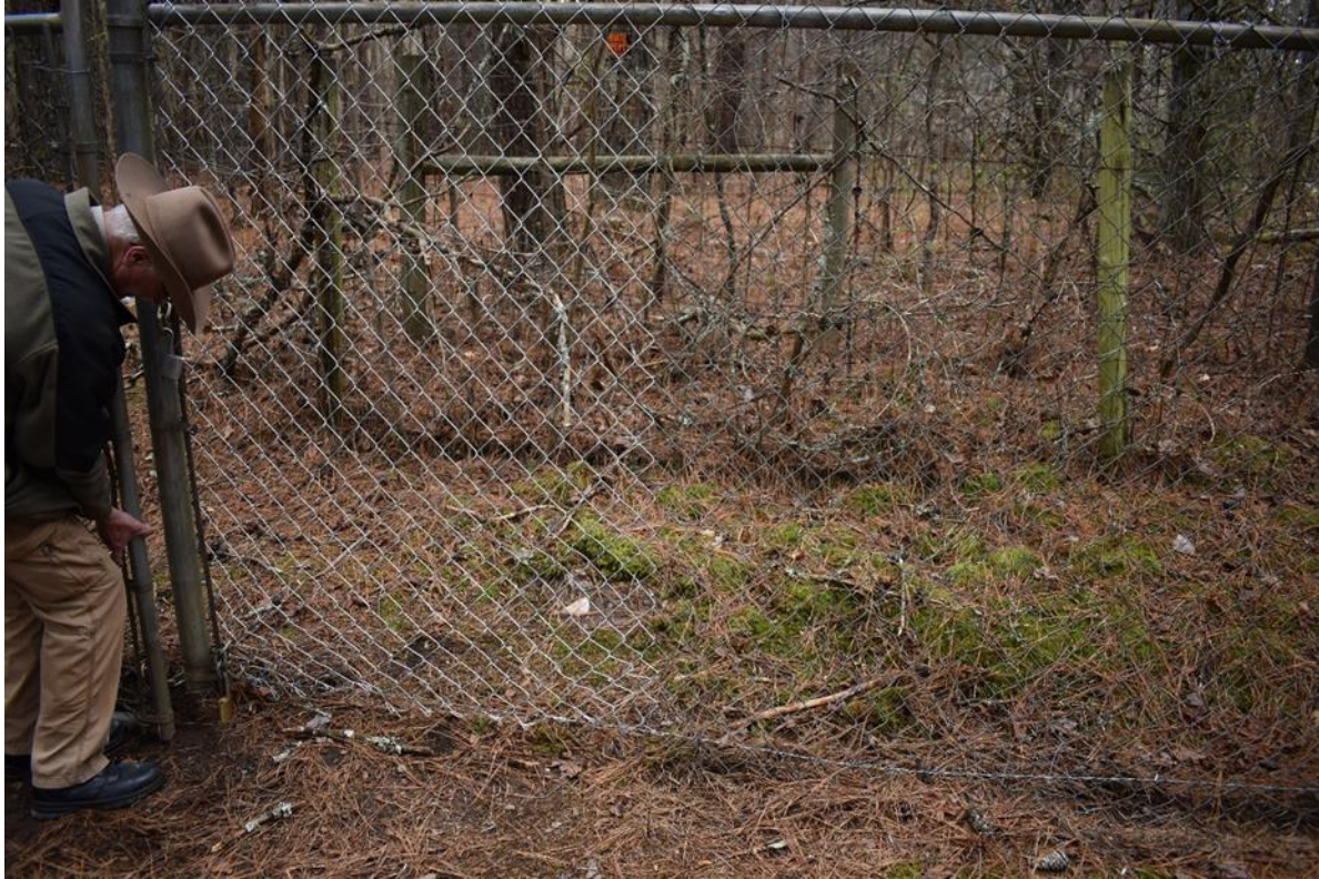
Figure 2. A photograph of repaired chain-link in the fence surrounding the former Hot Cell at the former Georgia Nuclear Aircraft Laboratory.
