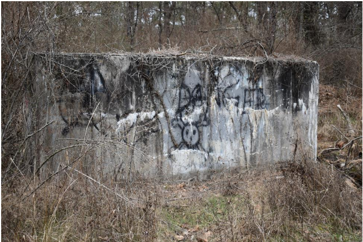
Figure 6. Graffiti on a low wall near an access road at the former GNAL site.
