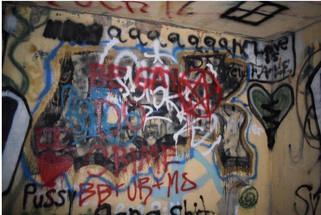
Figure 4. More graffiti from the pump station at the former GNAL site
