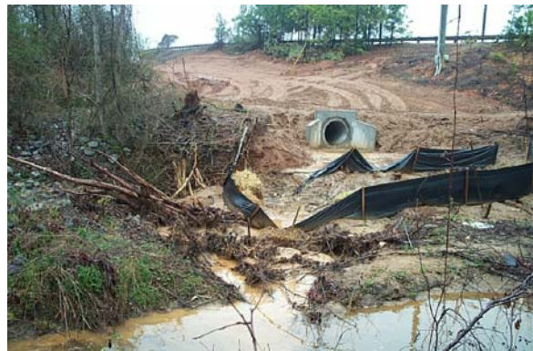
Fig. 1: Soil runoff near a fresh clearcut (Pratte)
